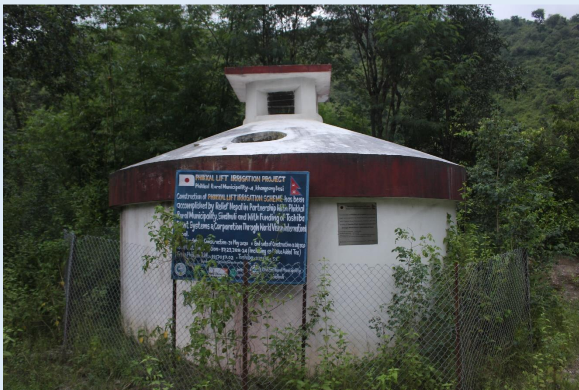
Photo 3: Water Tanks constructed by SIDS Nepal
